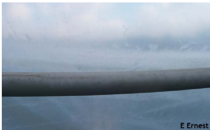
Greenhouse film around the PVC conduit with cloudy discoloration and signs of wear.
