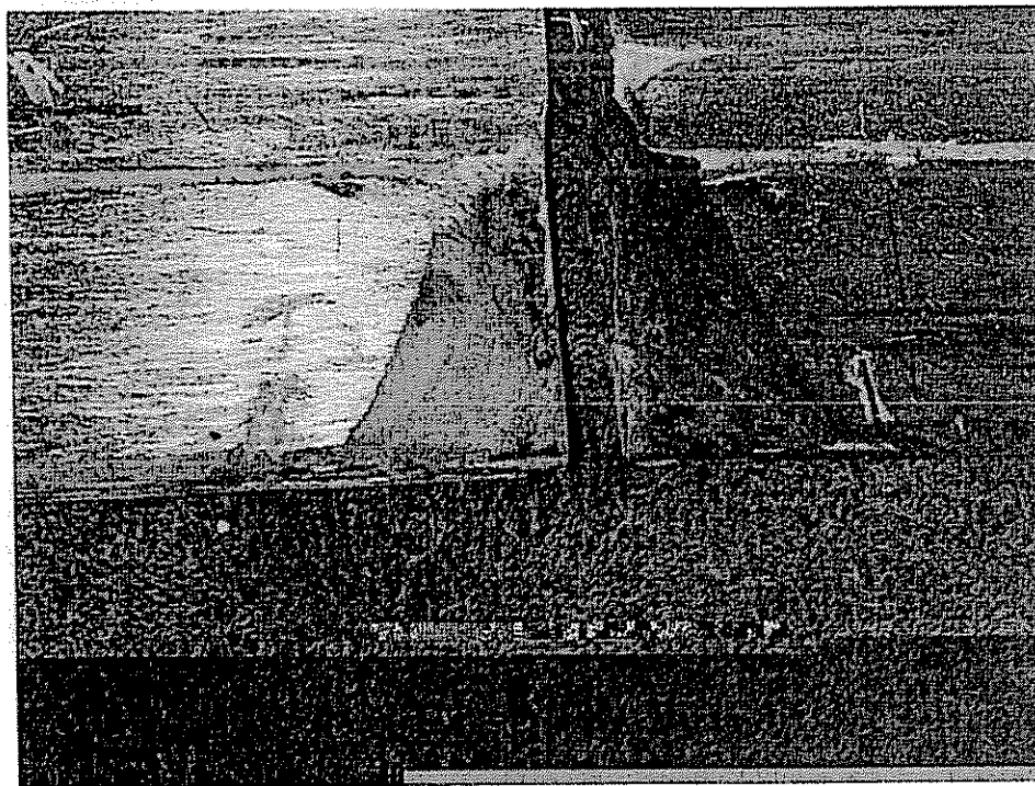
Figure 2.21 Corrosion at steel-composite interface at corner of sample TT-A.
