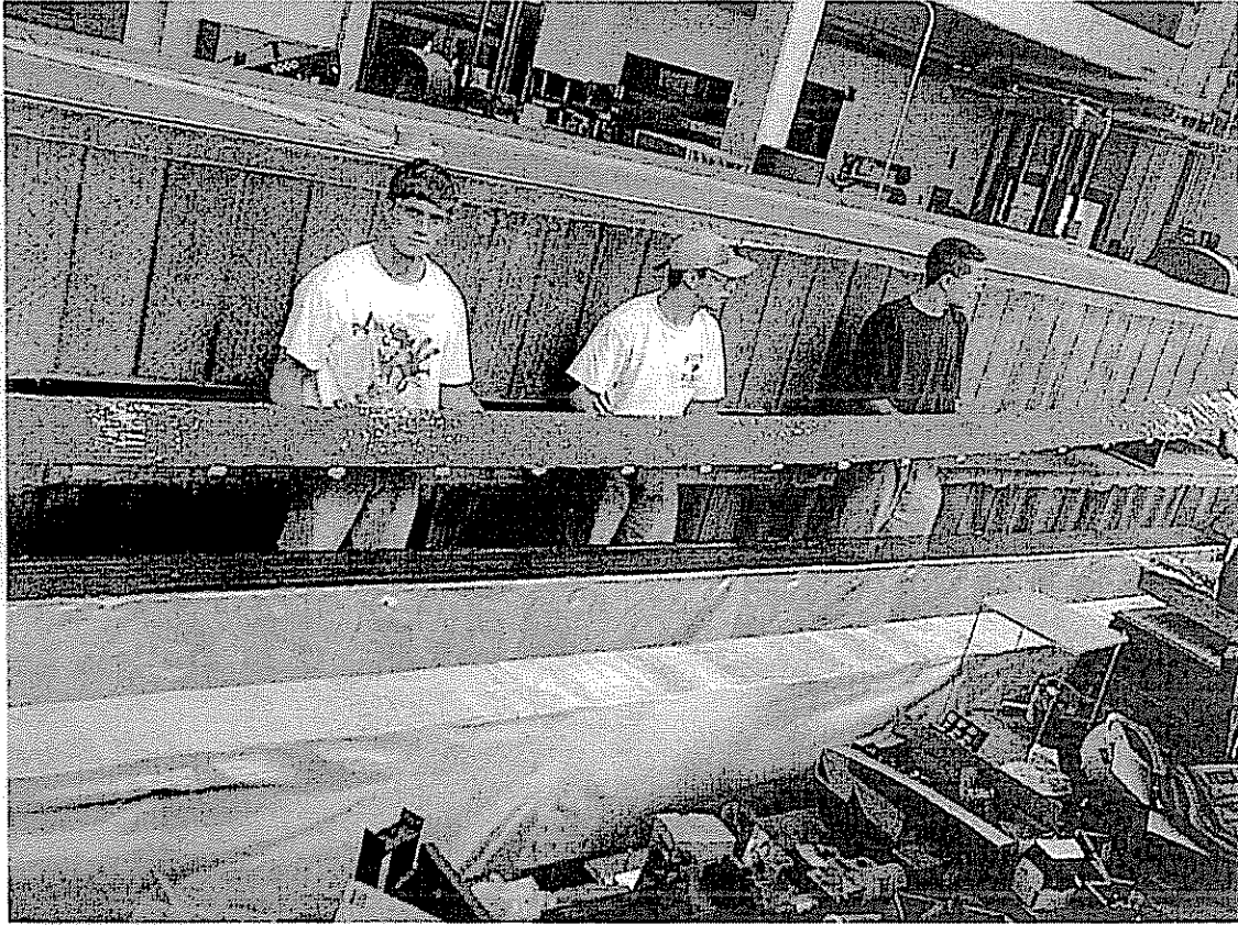
Figure 5.17 Lifting the composite assembly with full coat of adhesive prior to bonding to steel.
