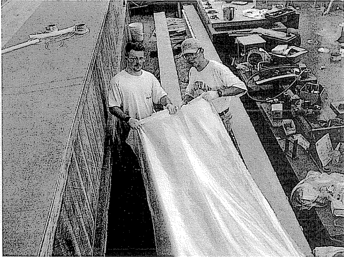
Figure 5.15 Pulling out 120-fiberglass scrim to place in bondline as a galvanic corrosion inhibitor.
