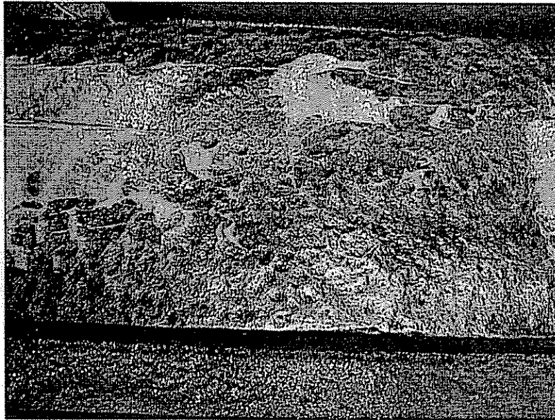
Figure 5.14 Pitted flange surface due to corrosion. Care was required to ensure complete adhesive coverage.
