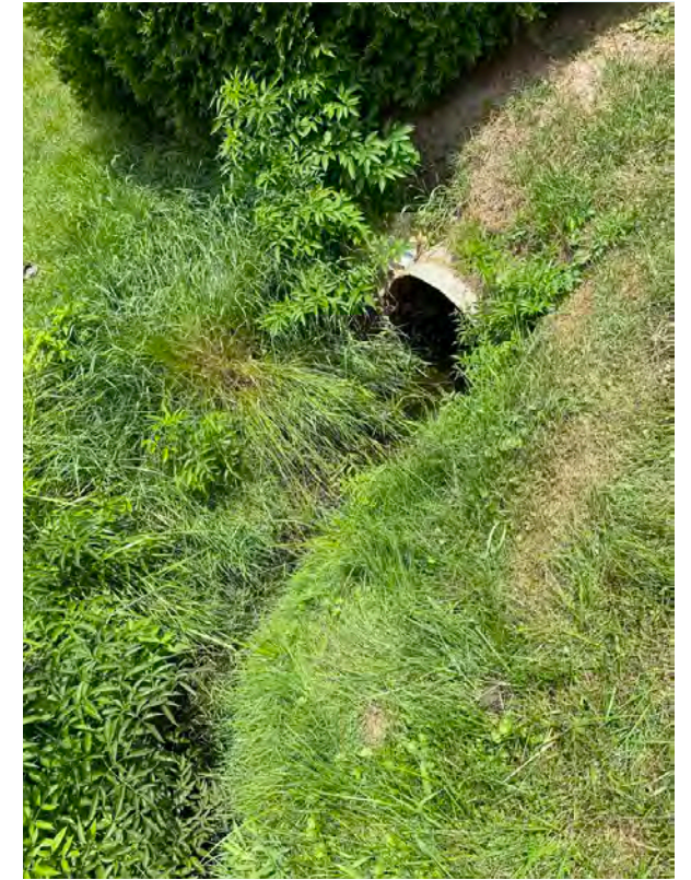
(right) Overgrown vegetation and sediment impede water flow from the ditch through shown culvert that leads to the Little Creek stormwater system.
