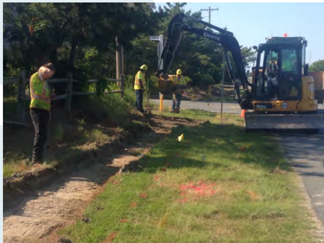
Excavation of one right of way bioretention area - photos courtesy of Delaware Center for the Inland Bays
